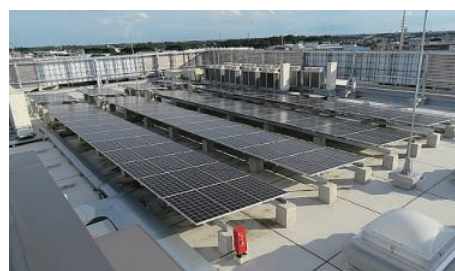
Solar panels of Tsuchiura Plant MI Building
